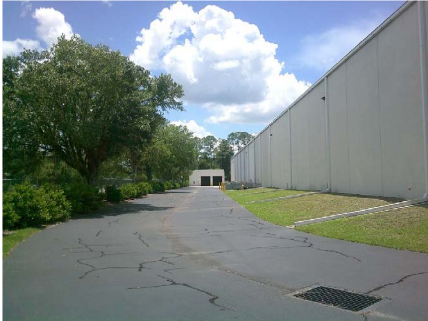
View of the north elevation of the building looking east towards the service garage. This is the addition added in 2011.
