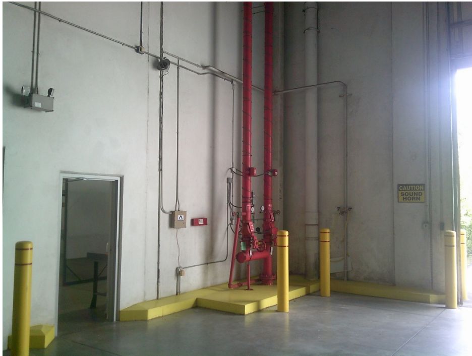
View of the fire sprinkler system.
