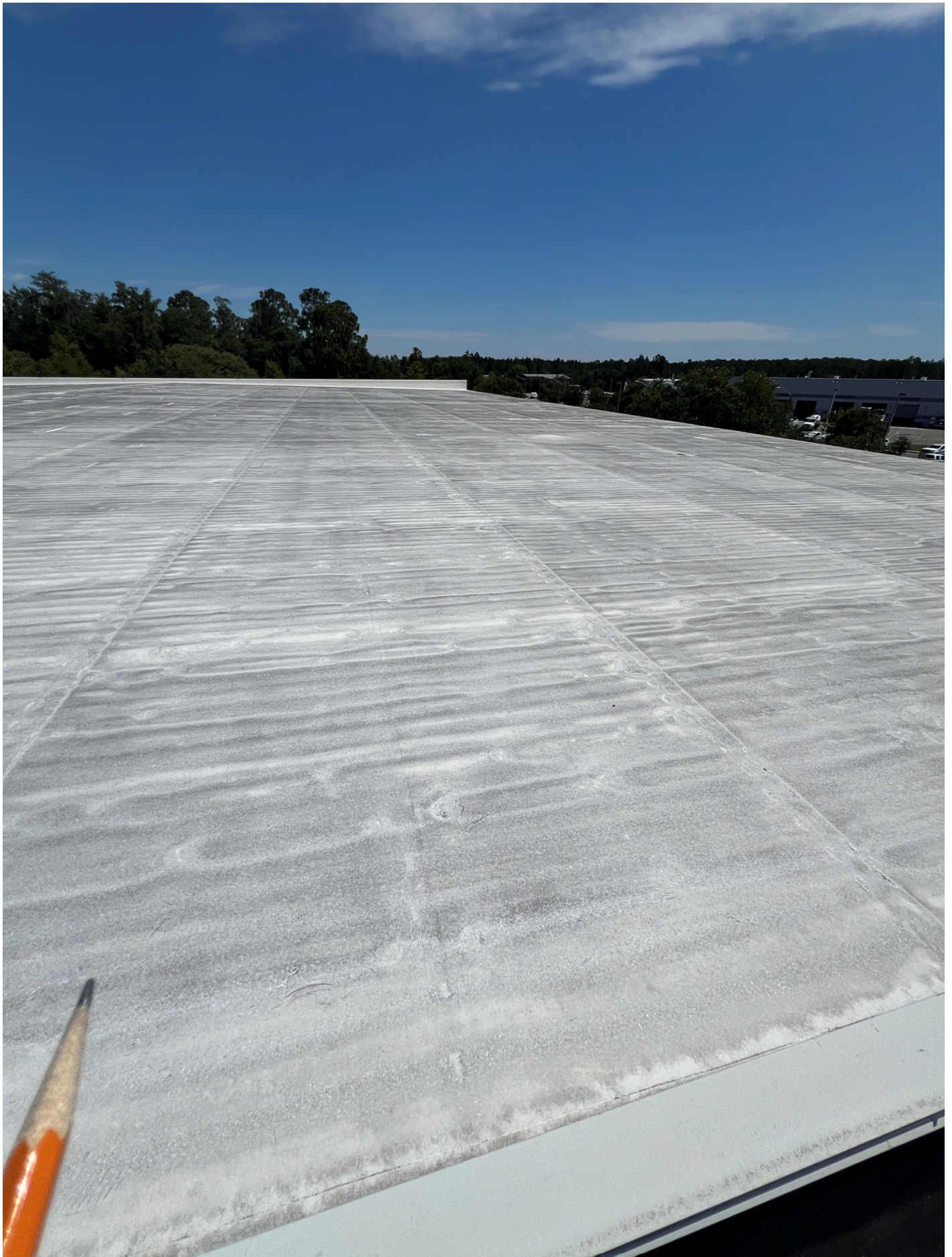
2011 warehouse addition single-ply PTO roof membrane, a few small vapor bladders
