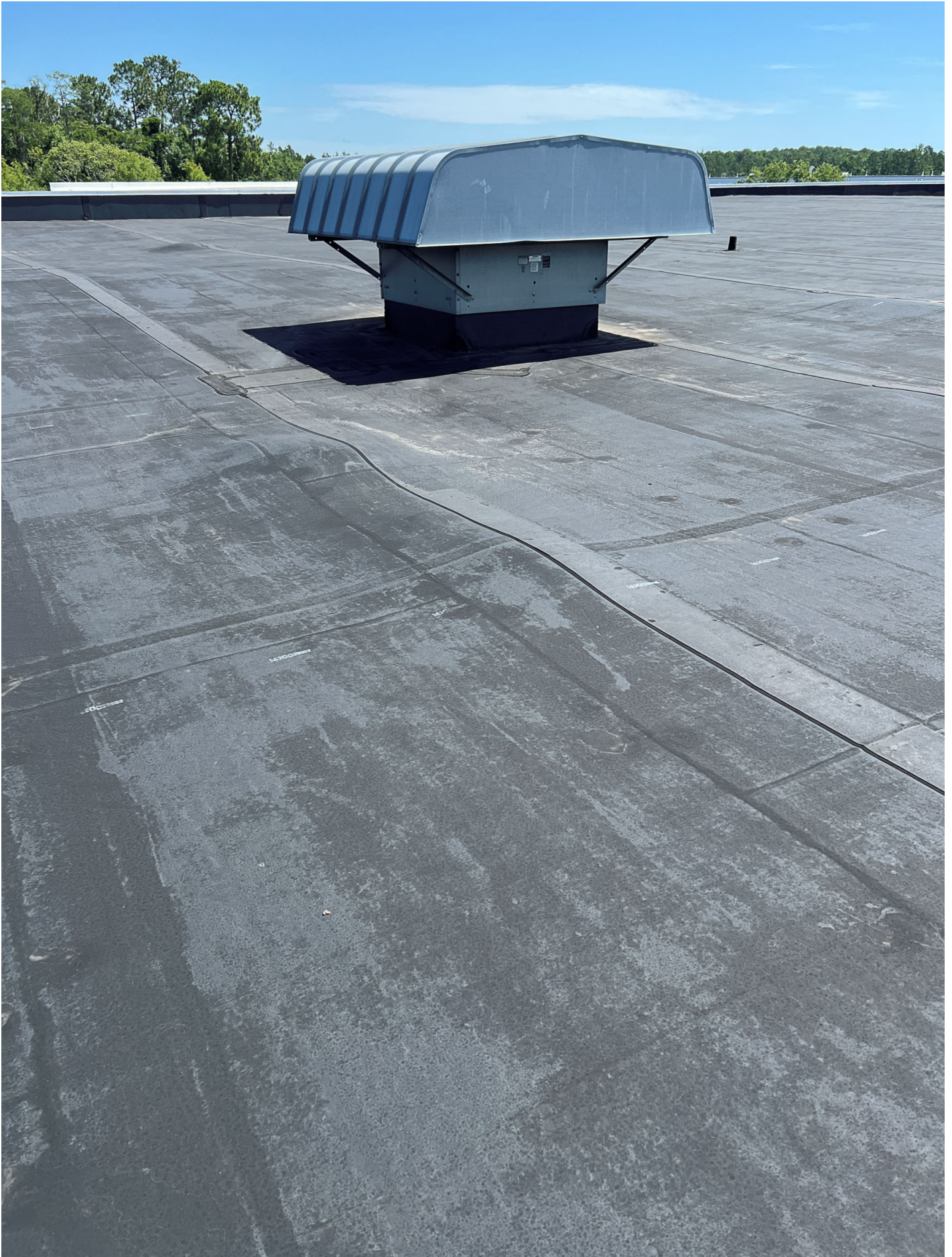
Large vapor bladders under the EPDM single-ply roof membrane
