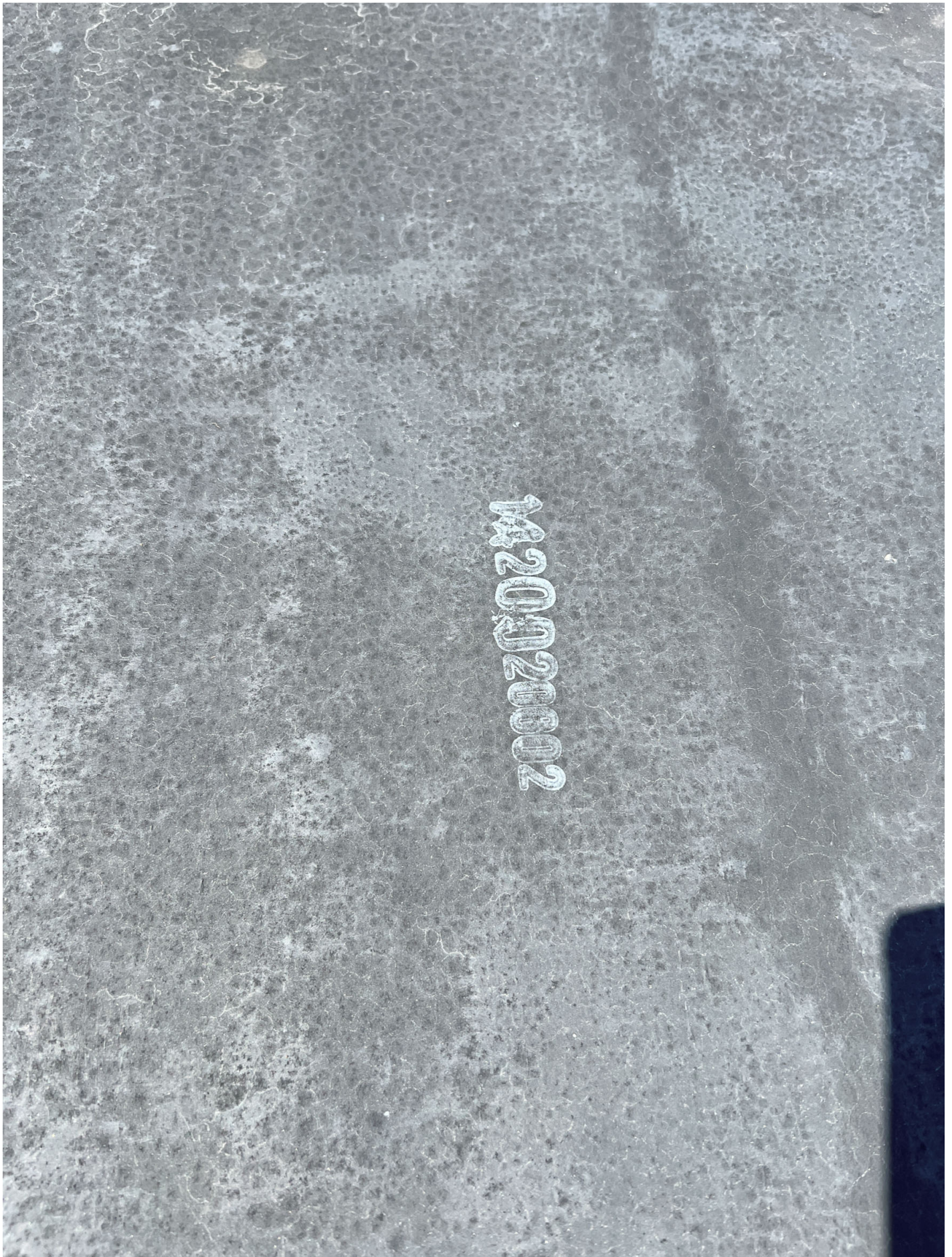
Admin roof area EPDM roof membrane breaking down from intense UV exposure
