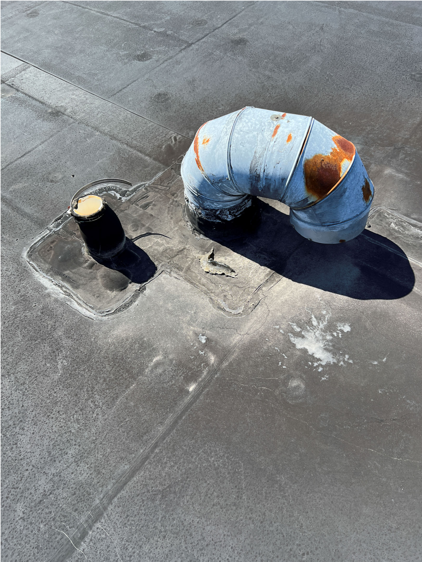
Lower Admin roof area previous patching
