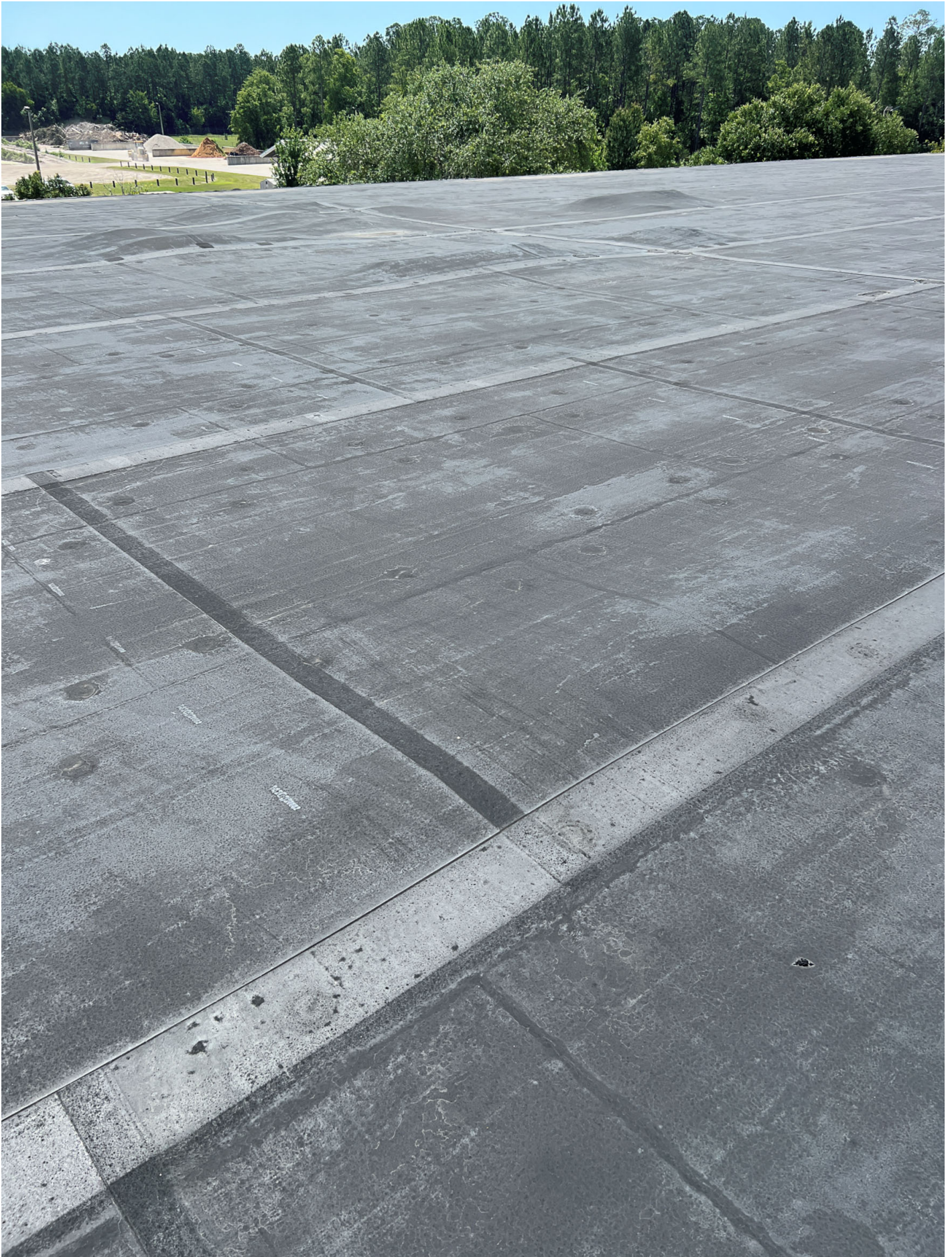
2000 warehouse roof open roof area with large vapor bladders plaguing the roof area
