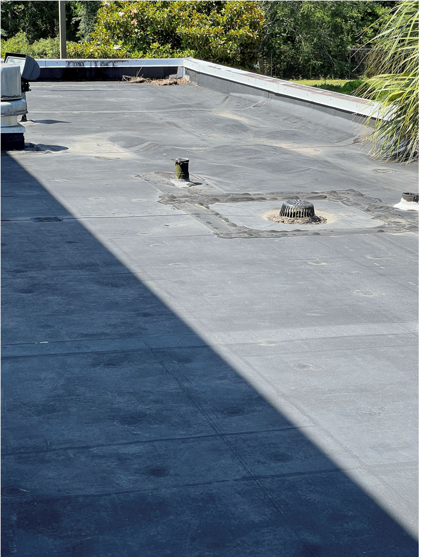
Lower admin roof viewing south large vapor bladders & patching
