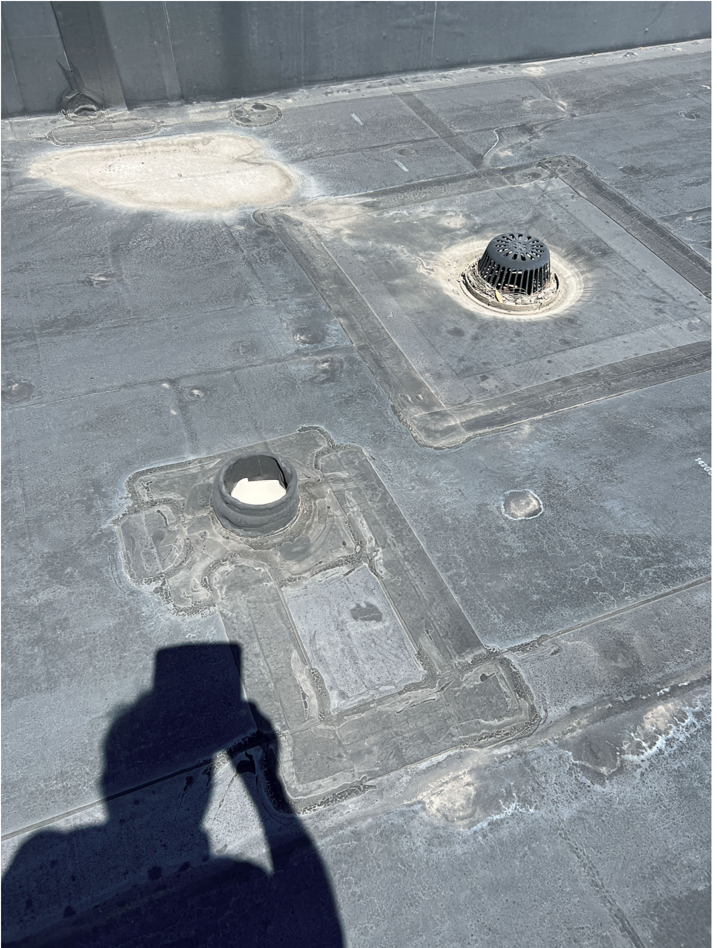
2000 warehouse roof west roof area adjacent to lower admin roof / roof drain & emergency o
