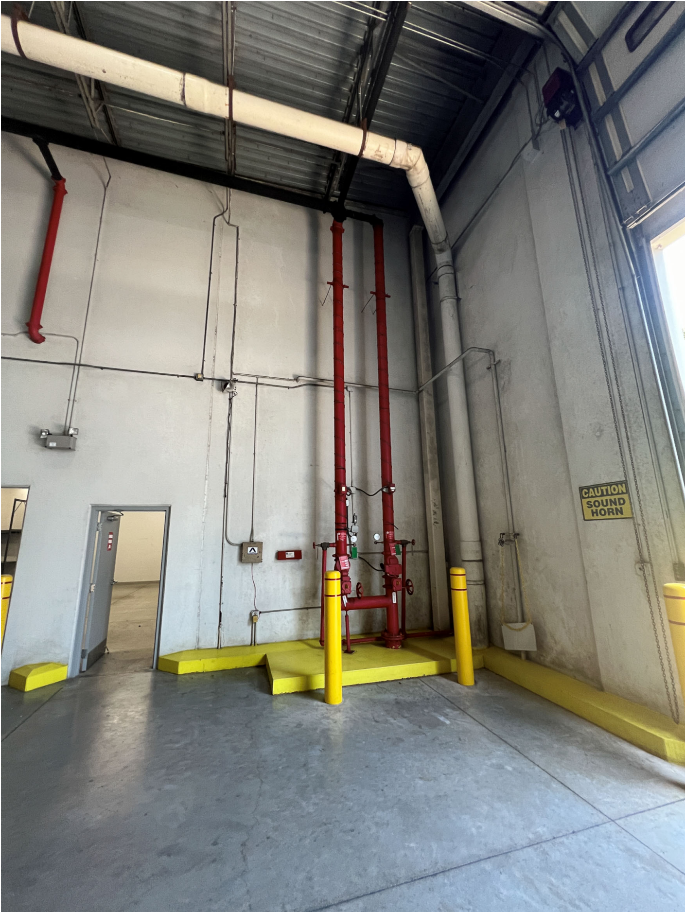
Warehouse fire sprinkler main
