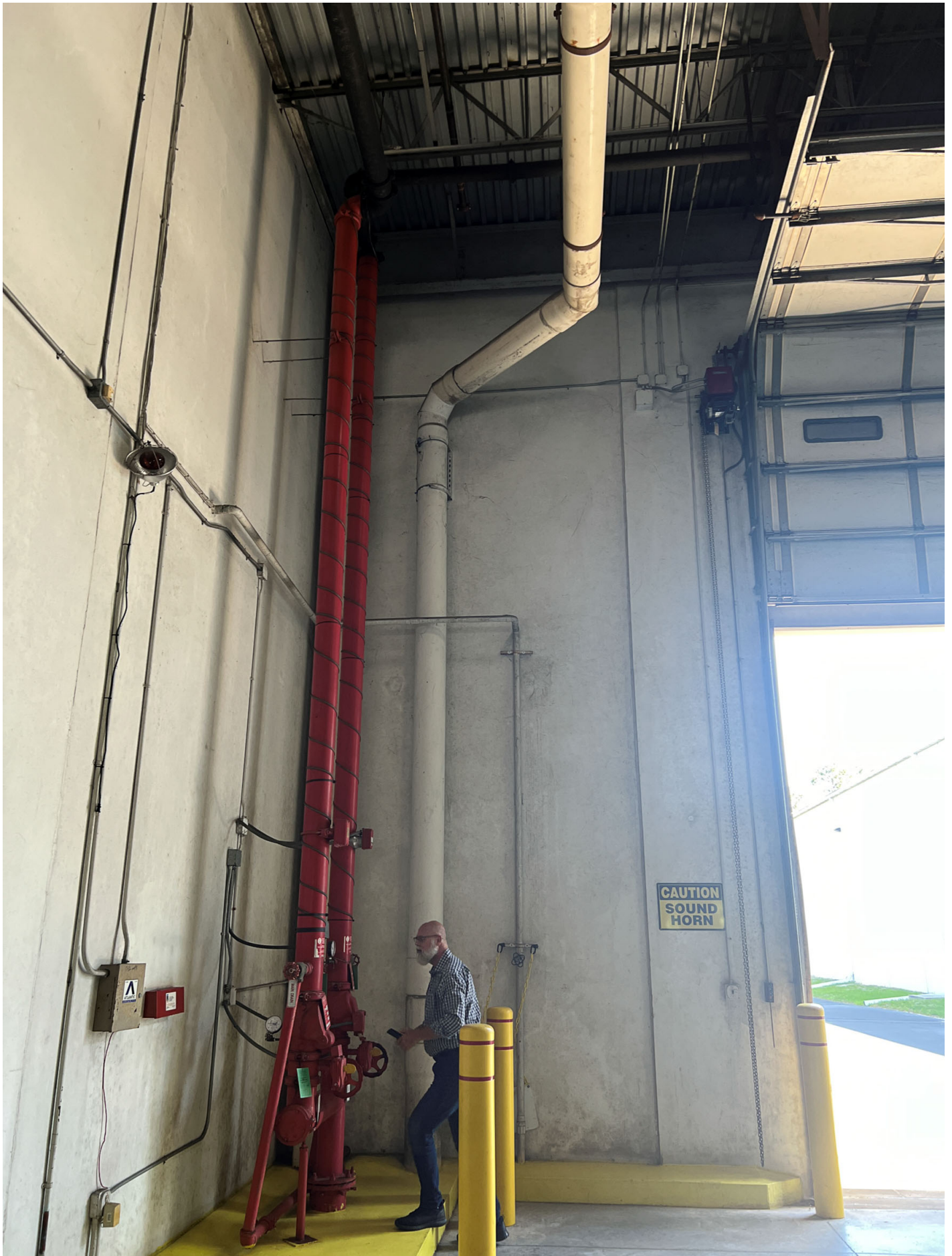
Warehouse fire sprinkler main
