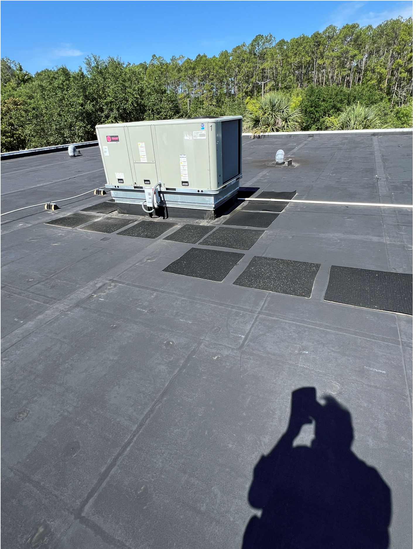
Admin area (lower) roof single-ply EPDM membrane w/ torched edges - one of four roof top
