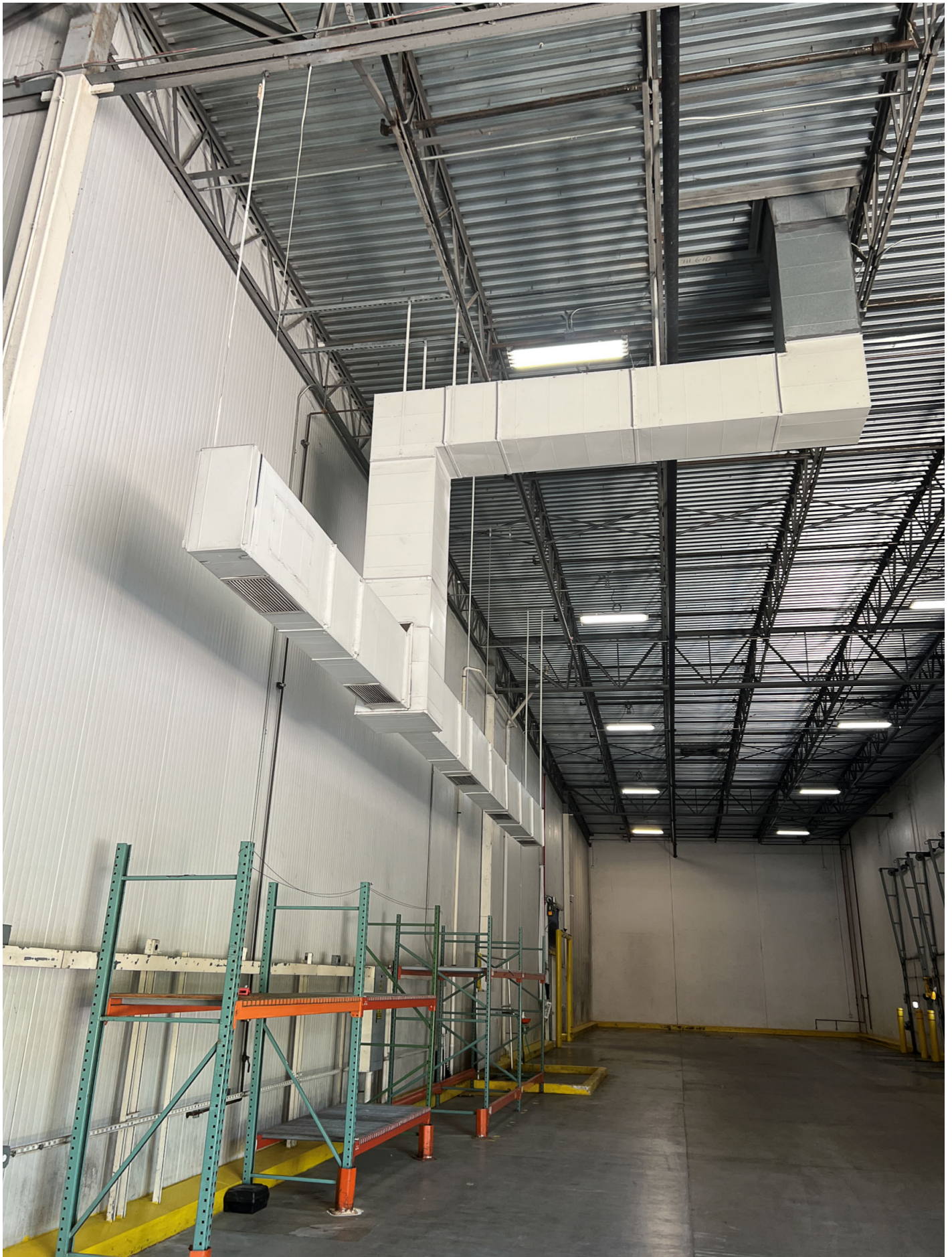
South storage / staging area for service truck loading at recessed loading dock
