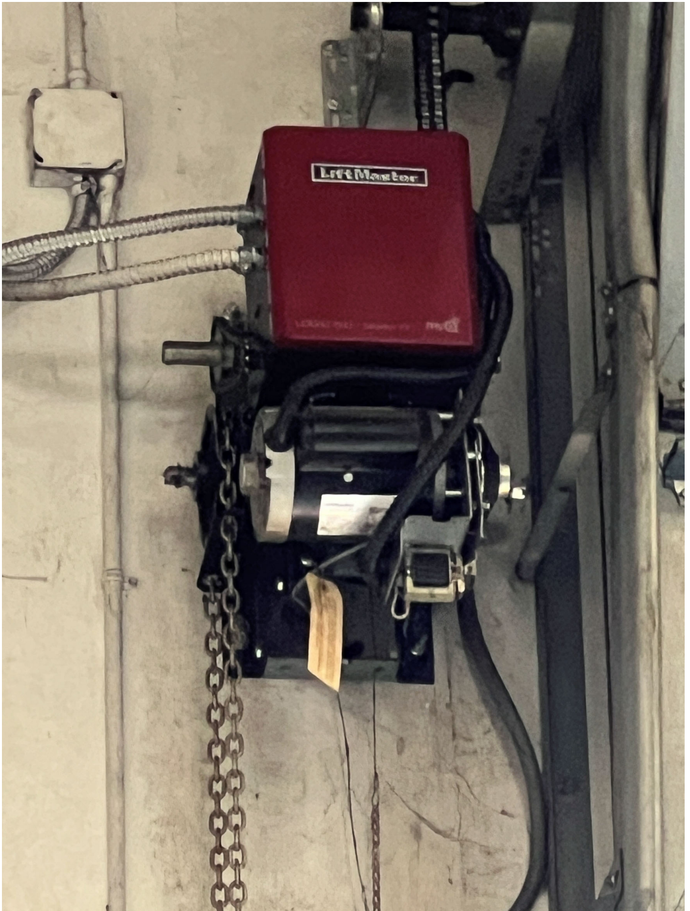
Motorized roll-up door operator - typical each door
