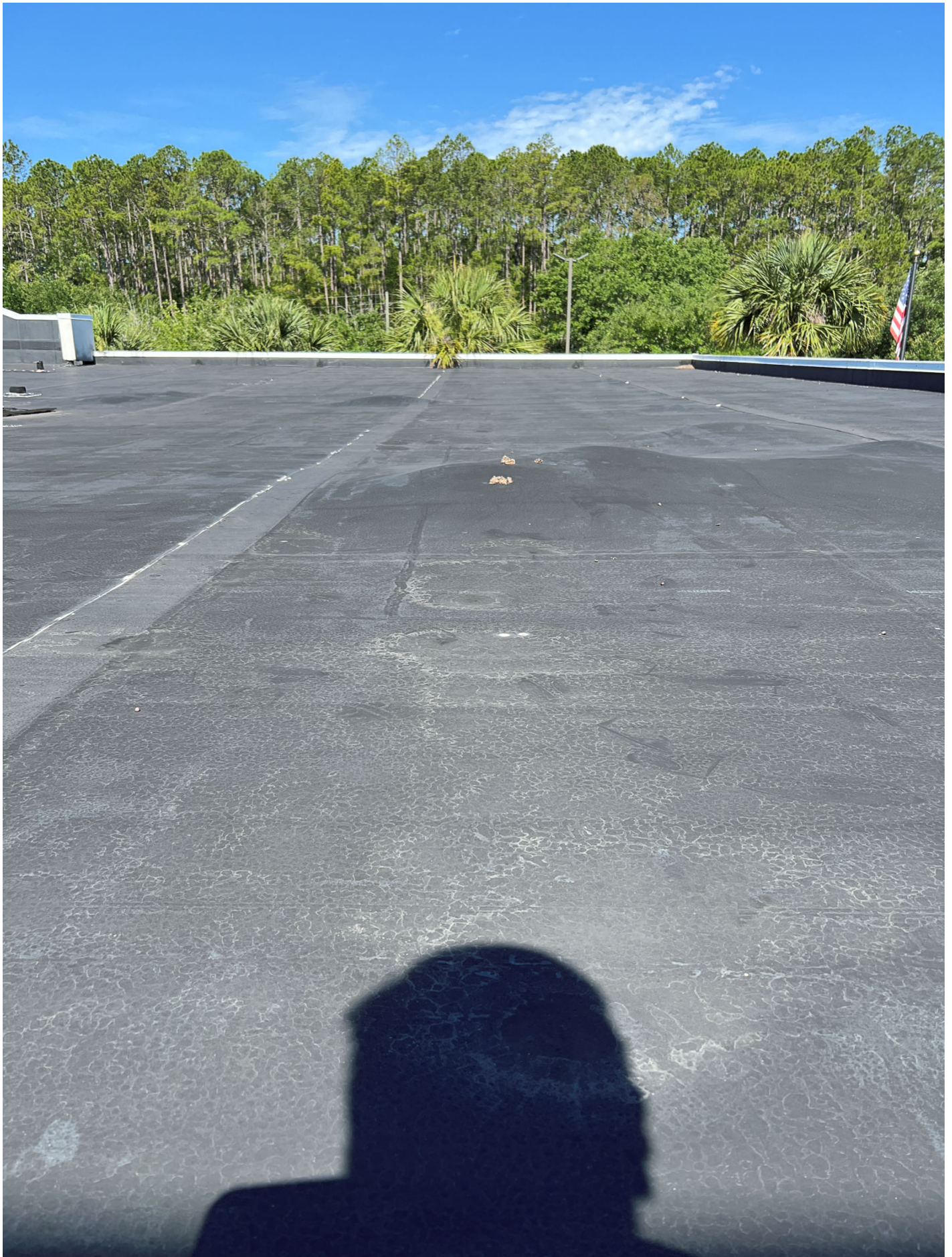
Open roof area with large vapor bladders scattered throughout the roof deck
