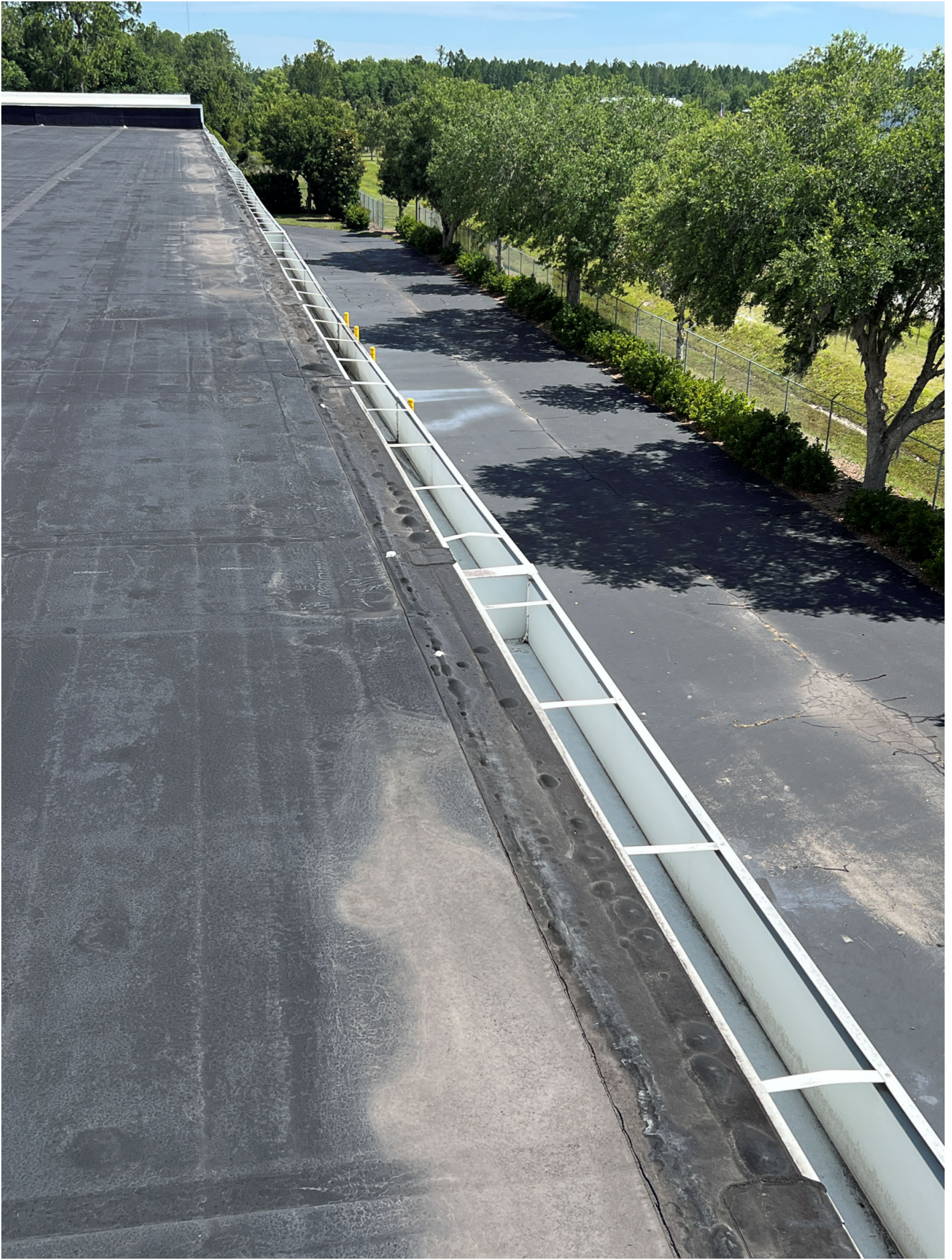
2000 warehouse east roof edge with gutters & downspouts / roof membrane deterioration
