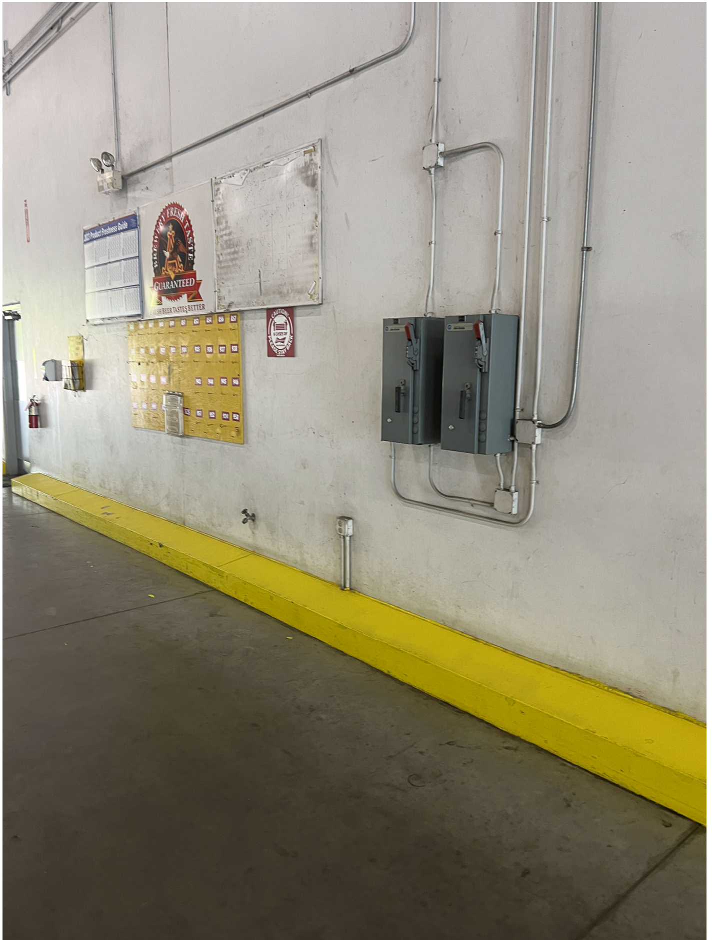
East wall of the west drive-thru bay - Emergency & general disconnects
