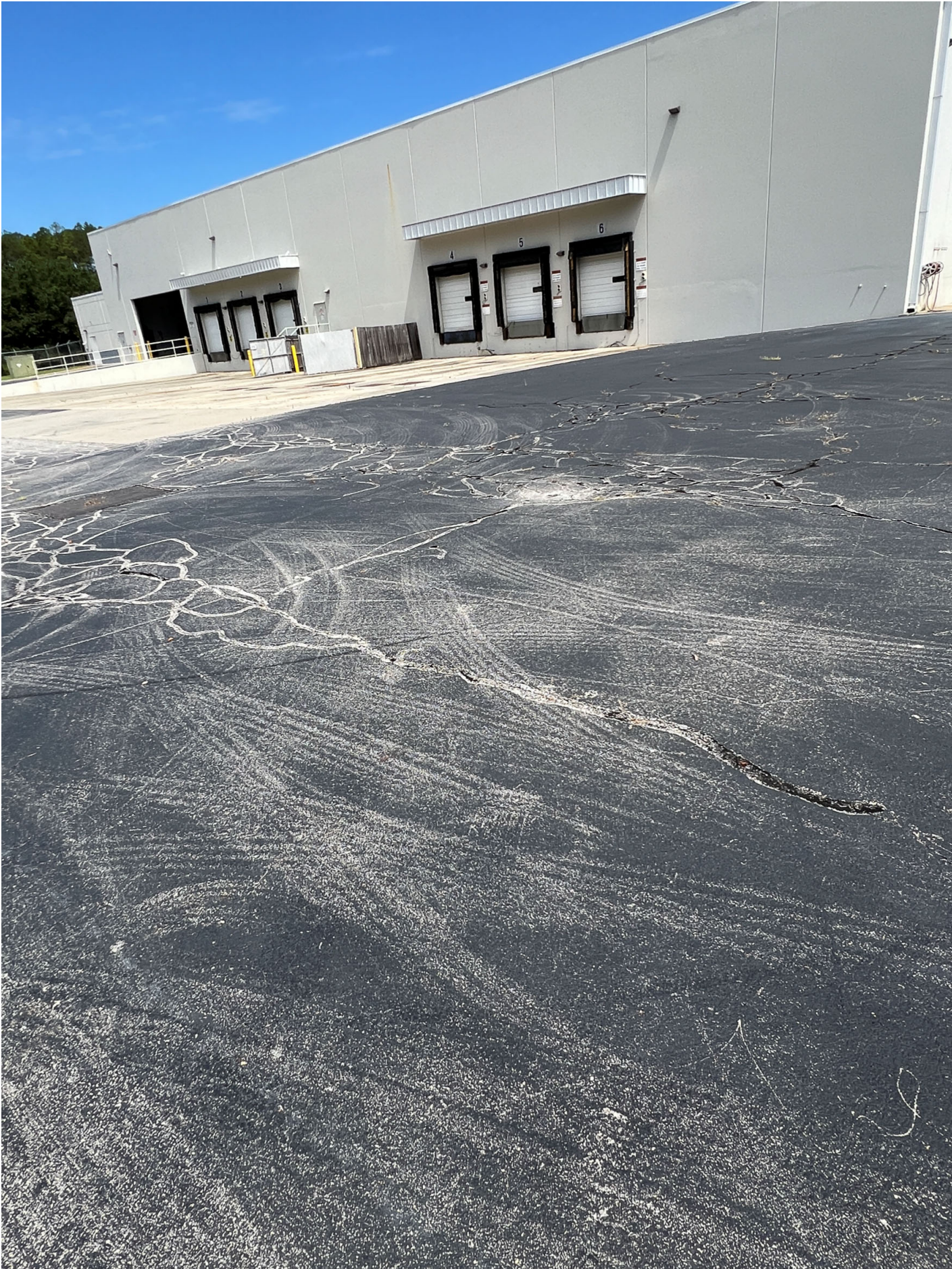
Southeast asphalt paved area requiring maintenance
