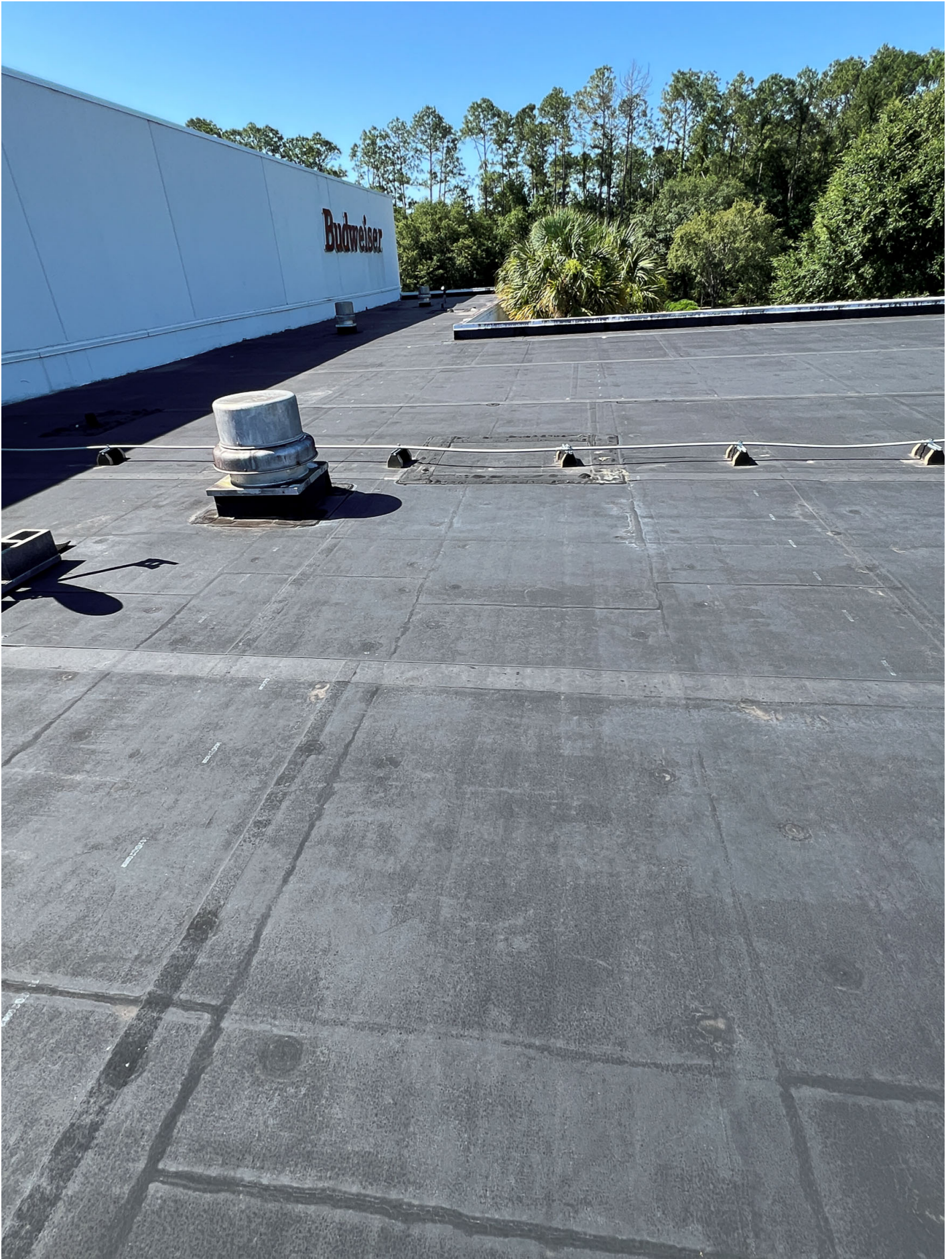
Admin area (lower) roof single-ply EPDM membrane w/ torched edges - exhaust fan on curb
