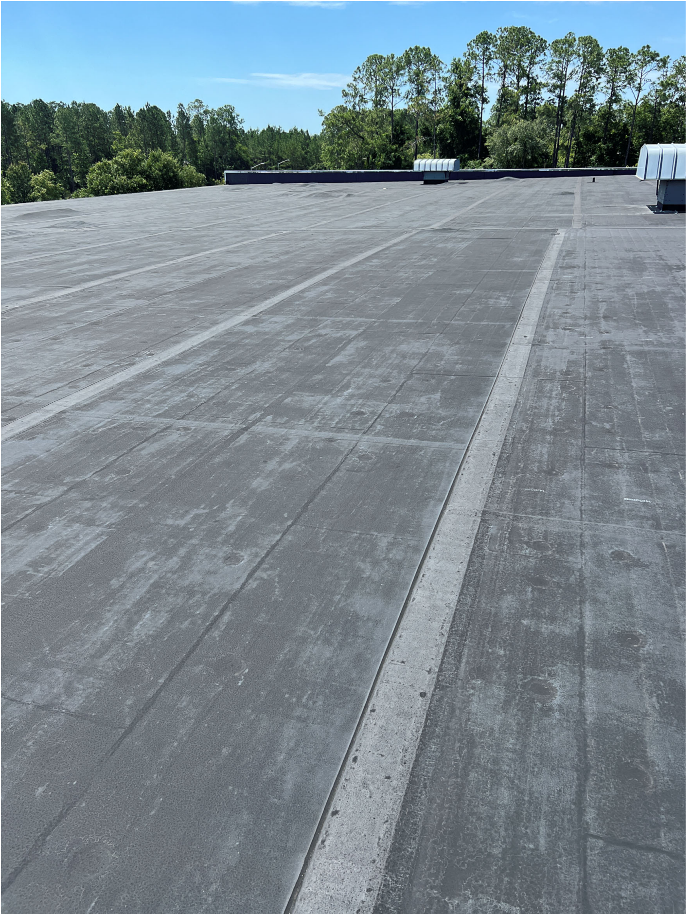
2000 warehouse roof open roof area with large vapor bladders plaguing the roof area
