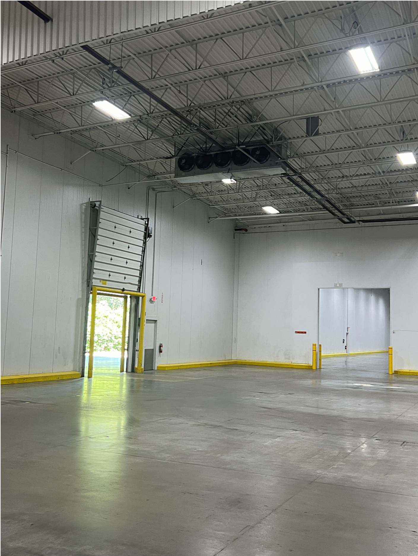
Central storage area with exposed utilities
