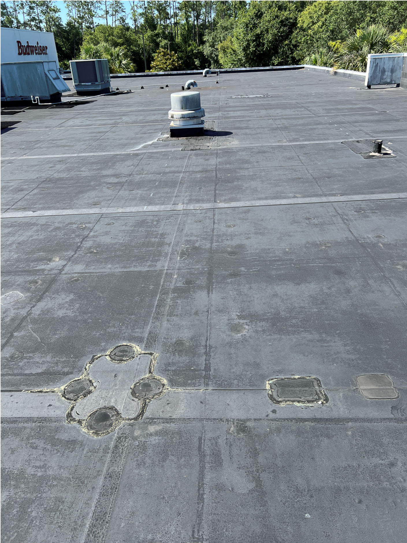
Lower Admin roof area previous patching
