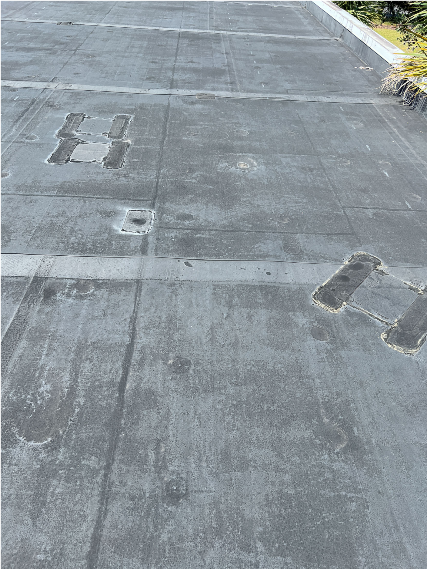
Lower Admin roof area previous patching
