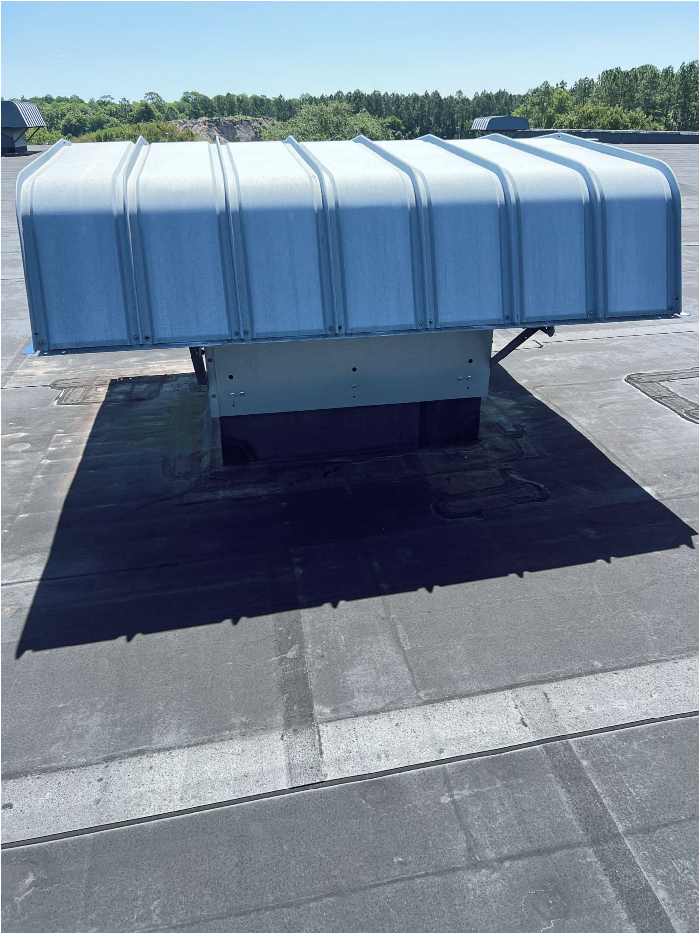
2000 warehouse roof with exhaust fan hoods
