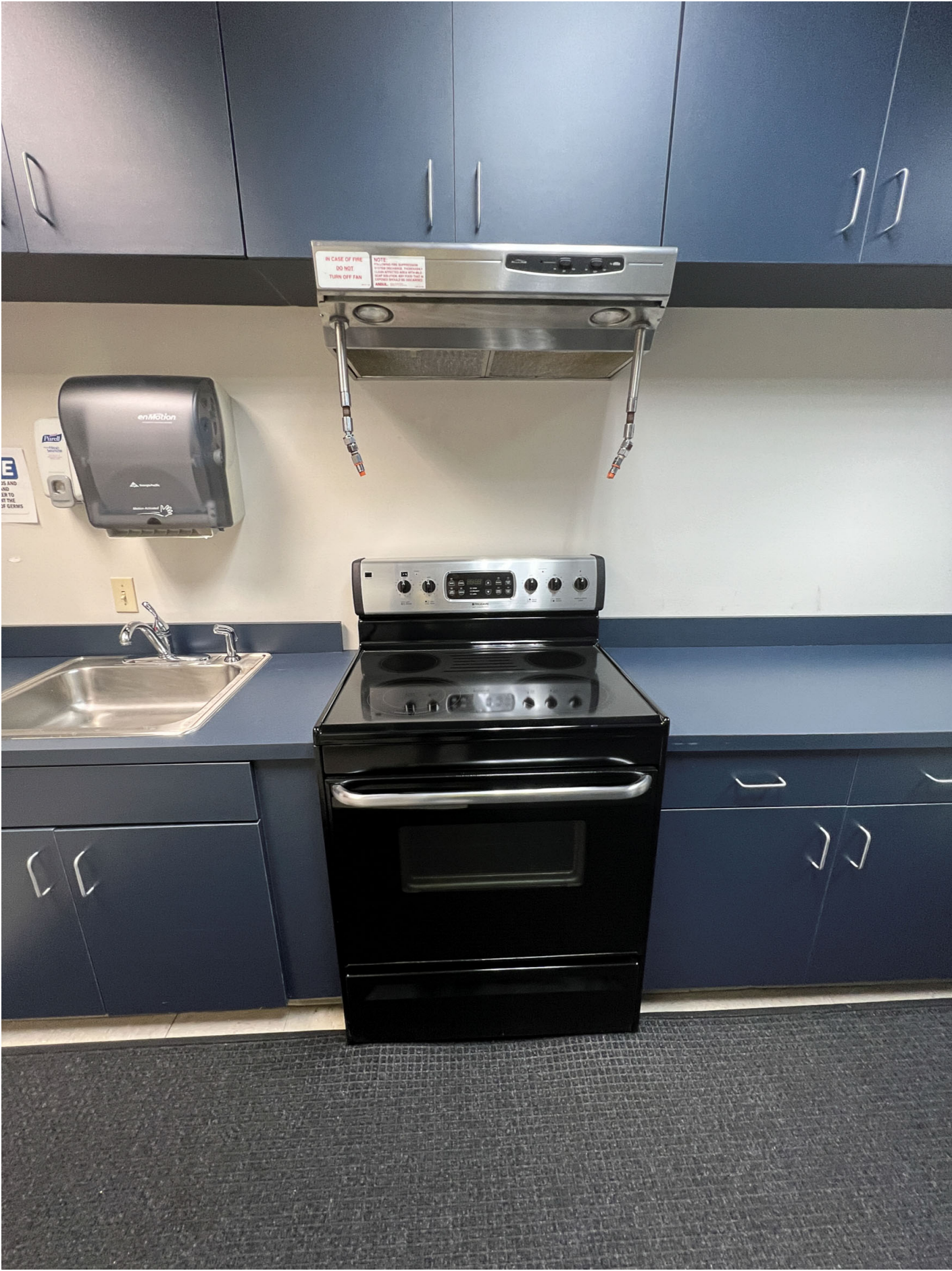
Stove / Oven with exhaust hood & Ansul system
