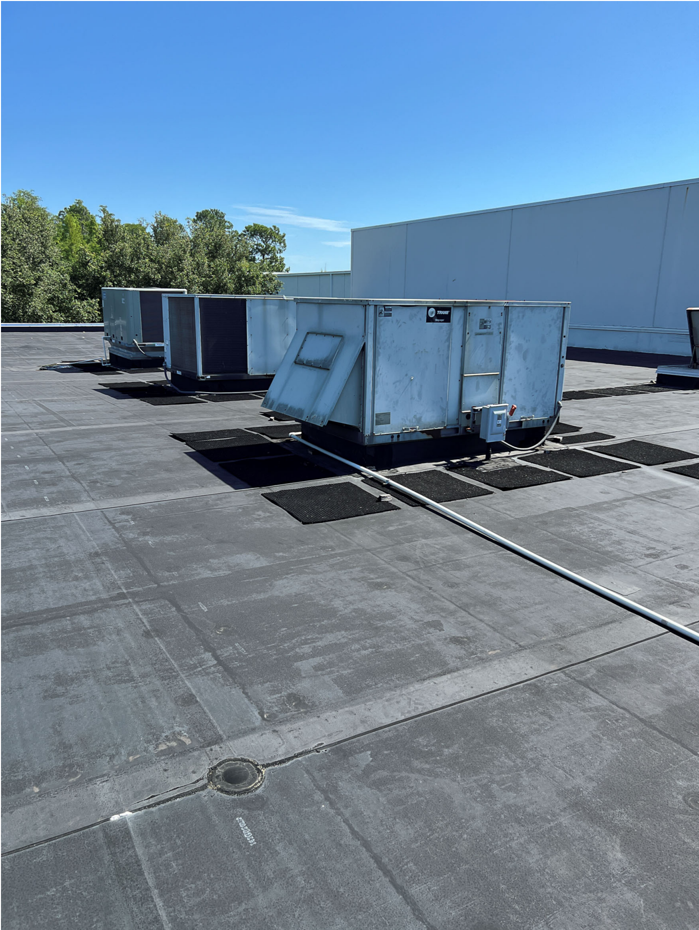
Lower admin roof area - Roof top A/C units
