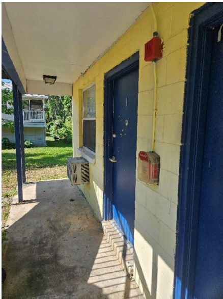
Figure 1: Typical exterior lighting fixture and fire alarm peripheral devices.
