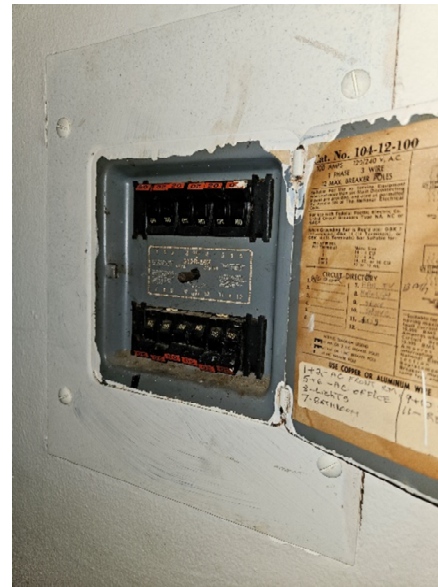
Figure 2: Typical unit electrical panel.
