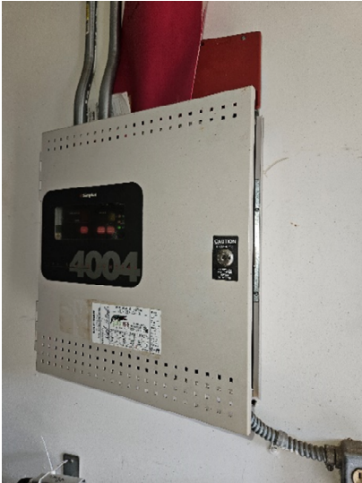
Figure 3: Cover of obsolete Fire Alarm Control Panel.
