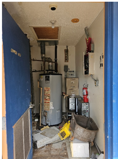
Figure 7: Hot water piping in boiler room
