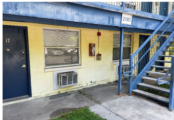
Figure 3: Damaged air conditioner
