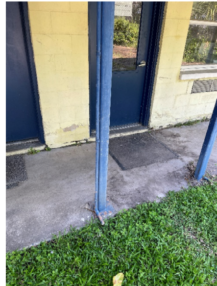
Figure 5: Condensate piping routed down support to grade
