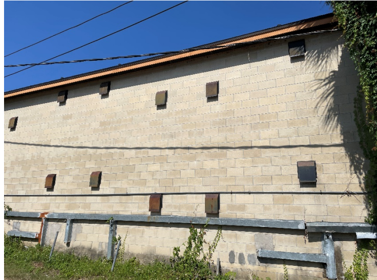
Figure 6: Surface mounted piping on building exterior
