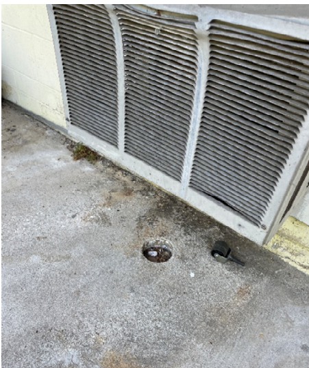
Figure 2: Damaged air conditioner and condensate dry well
