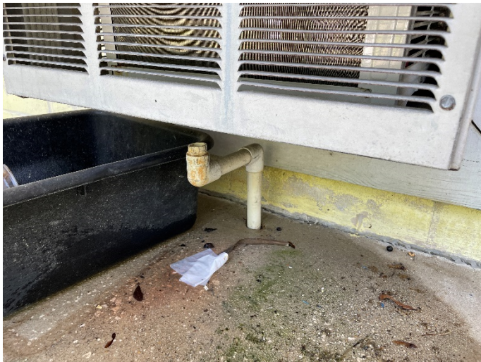
Figure 3: Disconnected condensate drain
